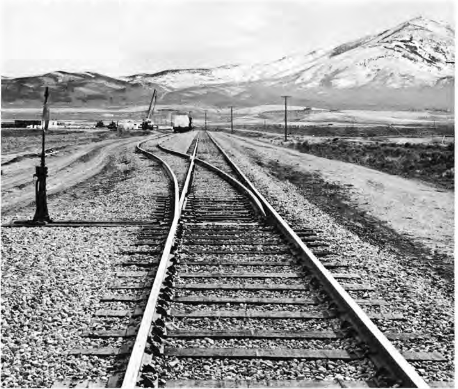
The completed track extension near the J. C. Penney site is opened and ready to serve the industrial park.
