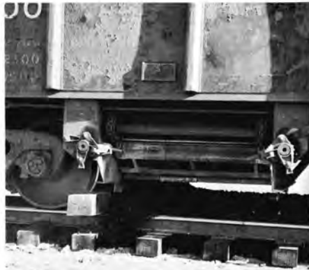
Tie is shown here 'plowing out' ballast during the "center dump" ballasting operations.
