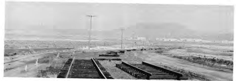
At railhead, "joint" ties are placed along the new right-of-way ready for the track panels to be delivered.
