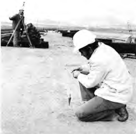
Engineer Tony Giovannoni and the surveying team set a "center line" for the new track.
