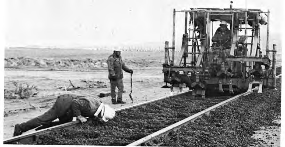
Track Foreman directs tamper operator to raise track and tamp ballast to ensure good track surface.
