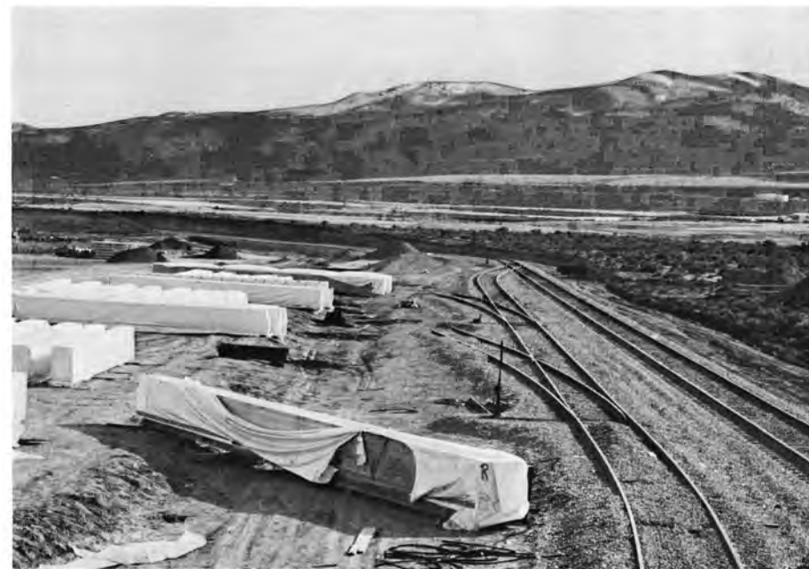
Photo shows the two switches from the run-around track that will serve the inside of the new warehouse. Also shown are rows of roof trusses that were unloaded from WP rail cars.
