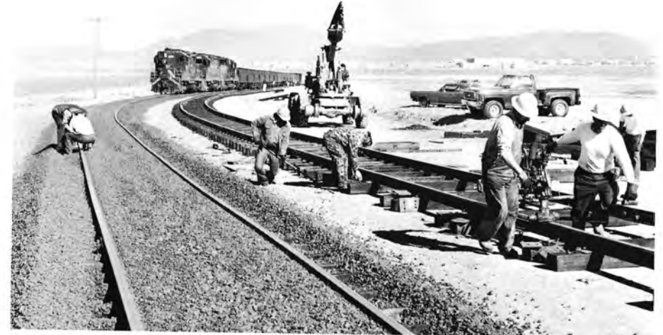
With ballasting operations concluded on main track extension, the track gang is rapidly assembling the new run around track adjacent to the construction of the new J. C. Penney's distribution warehouse.
