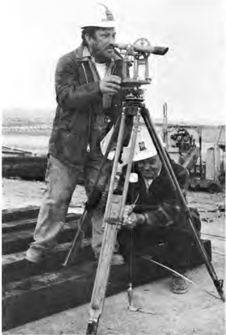
Surveying Engineer Ray Santiago, left, and Field Engineer T. G. Rutherford "stake out" the new right-of-way and set alignment stake for the new track.
