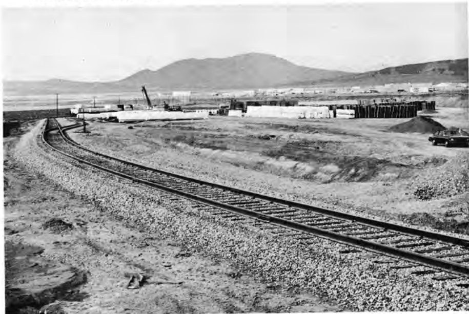
Following final rail aligning, tamping, and grooming operations, the new industrial line extension is complete and ready for traffic.
