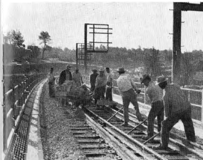
John Miller, section foreman (white hat with black band behind Nordberg spiker) supervises WP track workers installing guard rails in one of the final steps on the Feather River railroad bridge. WP expects to be running its trains over the new line in October. —Oroville Mercury photo by H. LeNair
