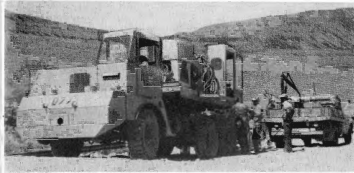
A Gradall excavator, one of the most versatile machines on the railroad, used for ditching, trenching, excavating, etc., and service truck with boom, welding outfit, drill press, electric grinder and tools. Picture was taken during job in the field.
