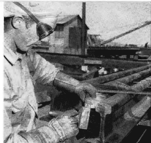
Just before welding, Don Kaufman cleans with solvent and files burrs off the rail ends.
