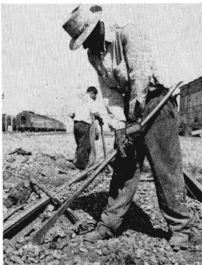
hands midway on the spike pulling tool, Duncan will avoid striking his hands on the opposite rail should tool slip.
