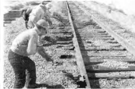
After new ties have been put in place, final phase is dressing the track with good ballast.
