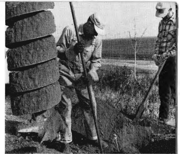
Above: Load of dirt removed from pole hole, on auger at left, will be used to fill second hole in which 8-foot-long anchor has been placed.
