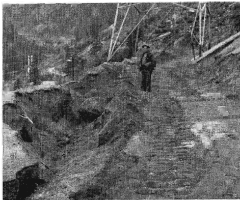
Engineer Inspector Lyman C. Landreth inspects area adjacent to PG&E roadway which crosses mountainside above top of the slide. Because geologists believe future slides may occur at this location, WP will tunnel under the slide.
