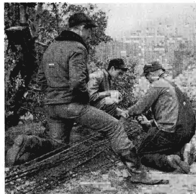
Bill Lake, George Hurley, and Lee Lawrence, Communications Gang No. 2, cut in phone to lines run around and above slide area. Clem Tomso, another member of the gang, is unseen behind Lee Lawrence.
