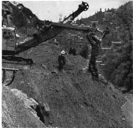
A Utah Construction Company engineer supervises excavation of dirt and rock from track area.
