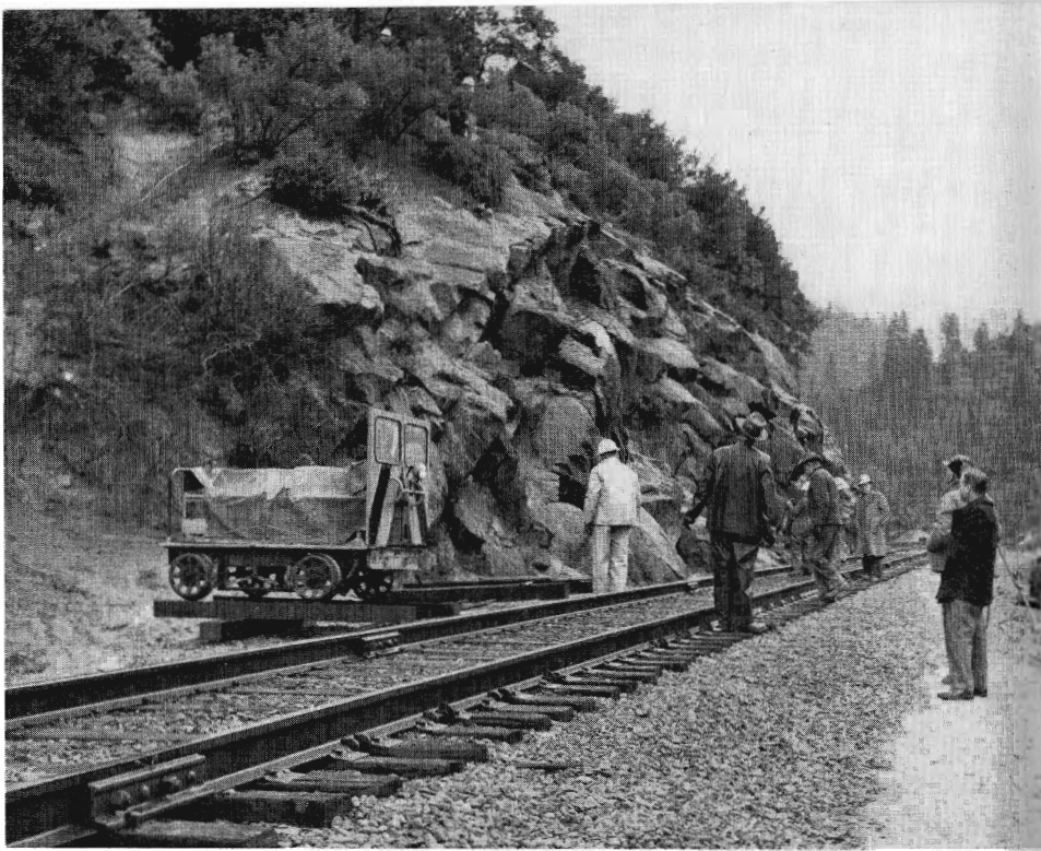
West entrance to proposed Tunnel 15 will begin at approximately this point, a great portion of which will be through solid rock. (See map on Page 11.) Completion is expected late this year.
