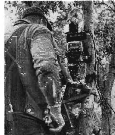
Lee Lawrence, telephone and telegraph maintainer, Communications Gang No. 2, tests telephone just installed on tree at top of slide. Instead of a bell, lantern flashes call men working at night.
