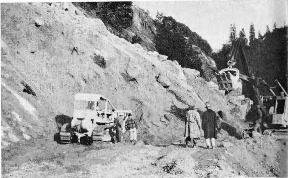
Picture above was taken December 28, by L. E. Hibbs, division agent and claim agent. Picture below was taken at same location on January 6. Work of clearing the slide area was most difficult during almost continuous rainfall and progress was necessarily impeded.
