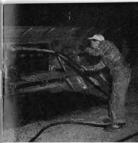
Frank Augait, electrician, hoses away dirt and acid which may have accumulated on batteries under diner.
