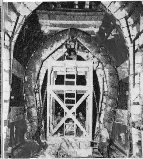
Closeup of collapsible steel form being moved with tunnel jumbo along track to new section. Lower portions of form will be spread out, when in position, to fit contour of tunnel walls.
