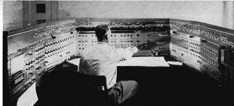
There are three control machines like the one above at Sacramento. On the top of the board is a miniature diagram of the section of track covered by one dispatcher. Small lights indicate the movement of trains.
