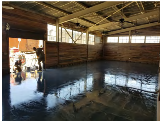
Museum Store floor completely primed on 6/22/21. Base coat will be applied next.
