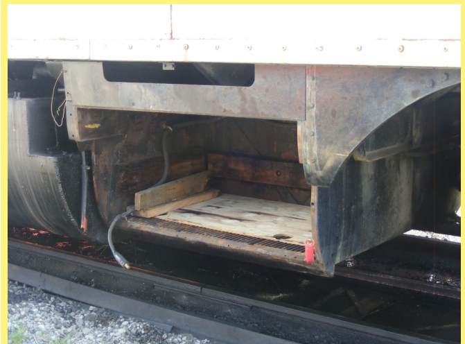
WP 917's right side battery box, prior to cleaning. Regular cleaning helps slow the corrosive effects of battery chemicals on the metal of the locomotive. The wood lining prevents terminals from inadvertently touching the metal body.
