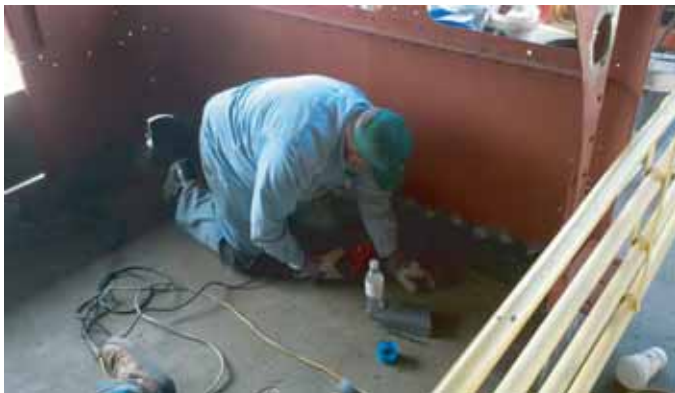
Dick Coudin drills holes for rivets at the base of the cab.
